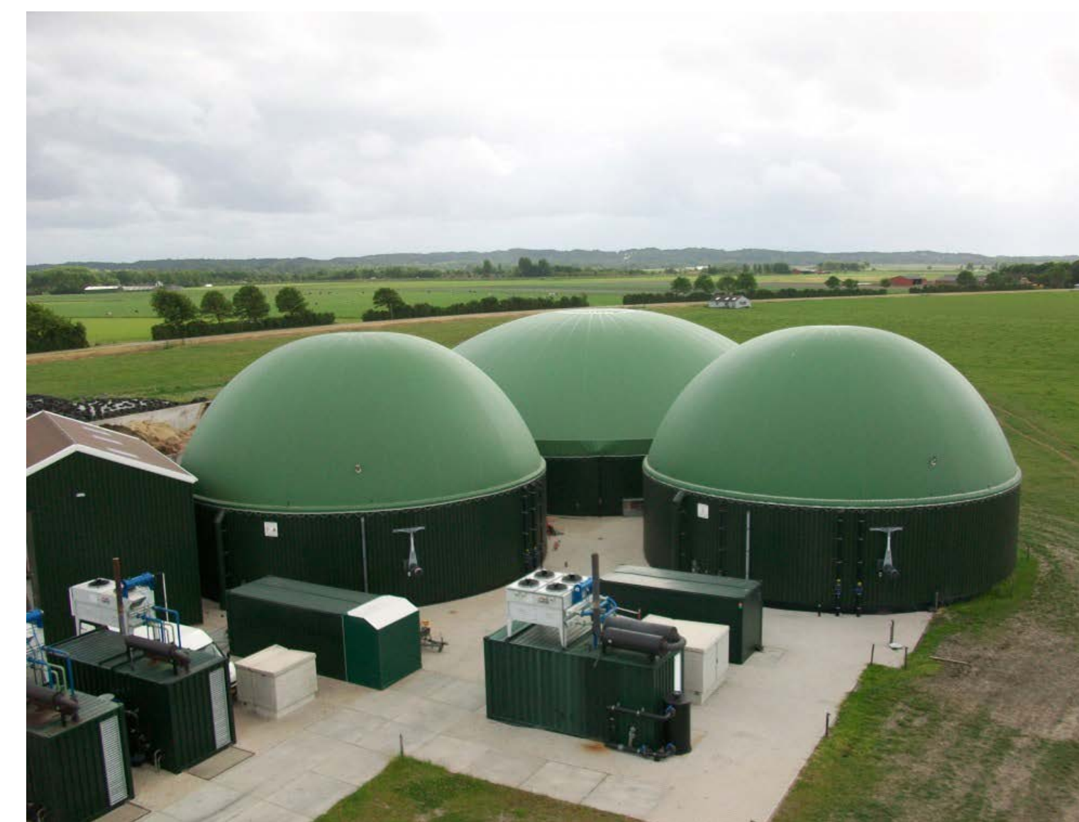
Figure 3. Operating Anaerobic Digester Site
