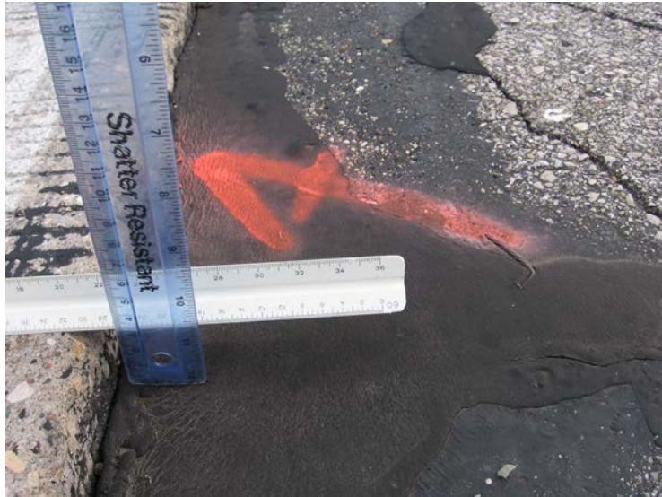
Figure 4. Lane to shoulder drop off in test section of RCA/5 (I-35 in Hamilton county mile post 131.40 to 131.45).
