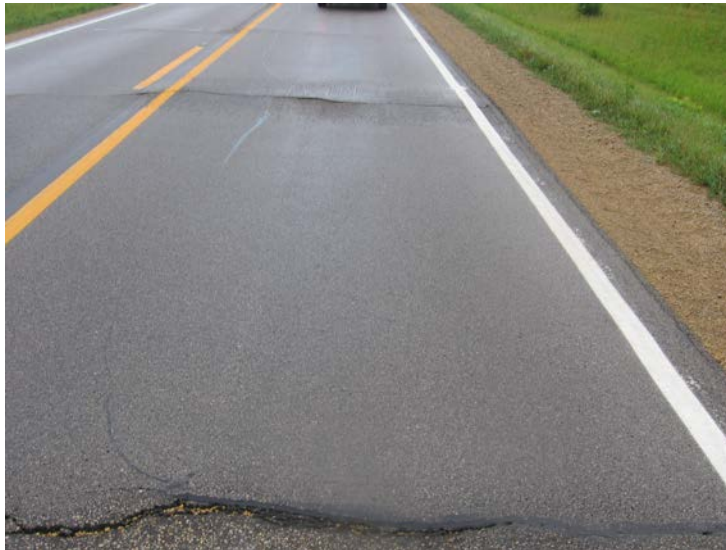
Fig. 9. Picture of reflection cracking on AC-overlaid virgin PCC pavement (No. 6: IA139 in Winneshiek County)
