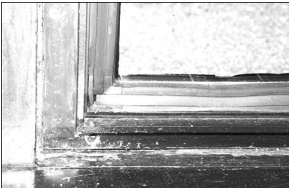
Fig. 14. Closeup of rust on interior face of frame, broken screws, and new gasket, 2008 (Photograph by Robert Whitehead).
