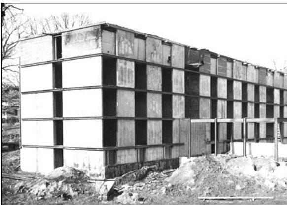
Fig. 6. Crawford Dormitories, 1953, Eero Saarinen & Associates. Dorm under construction showing precast assembly system (Presidential Files, Special Collections, Cowles Library, Drake University).
