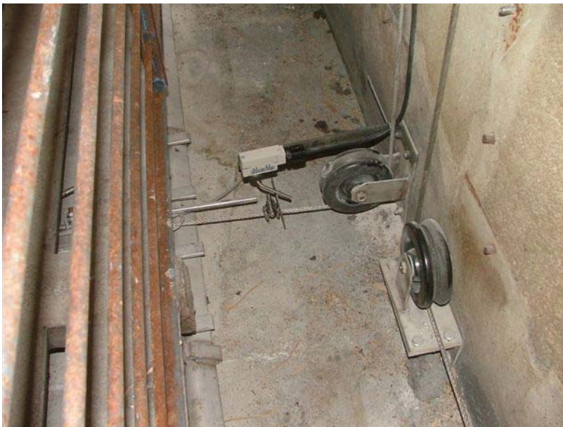
Photo 4. This scraper system showing pulleys with cable leading to the motor.
