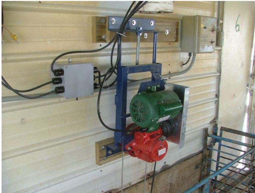
Photo 5. Safety features of the scraper system above the floor.
