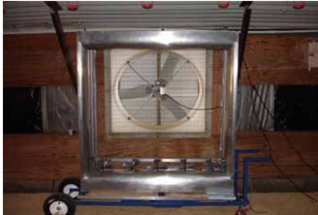
Figure 3: Fan assessment numeration system (FANS) unit being used in the Tyson Study to find the ventilation curve of individual exhaust fans.
