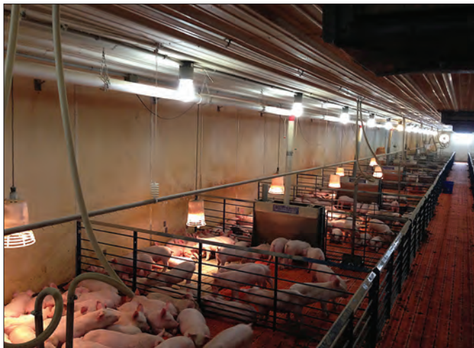
Figure 1. A swine nursery with the electrostatic system mounted on a pipe.
