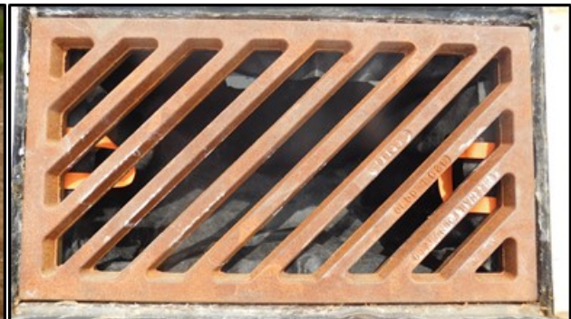
(f) catch basin grate
