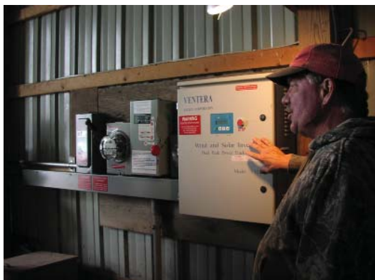
Jack Bensink explains the combined solar PV/small wind inverter installed on his farm with partial funding from a Farm Energy Working Group mini-grant.
