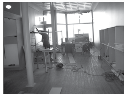
A mid-construction view of the new Lakeshore Museum Center Archives reading room.
