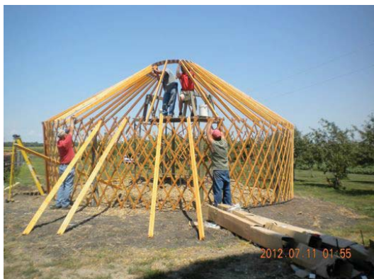
A wooden lattice (part of the kit) was erected to frame the perimeter wall. Wooden rafters (approximately every 2' on lower wall) formed the roof.
