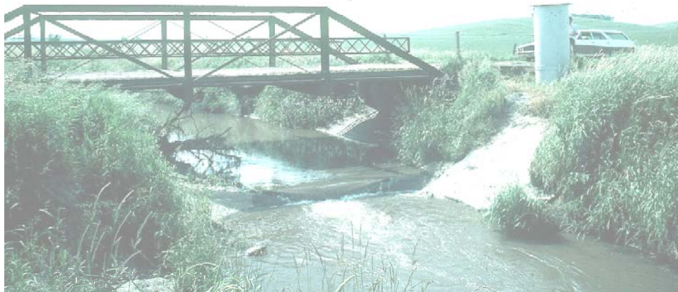
Figure 1. An automated surface water quality monitoring system
