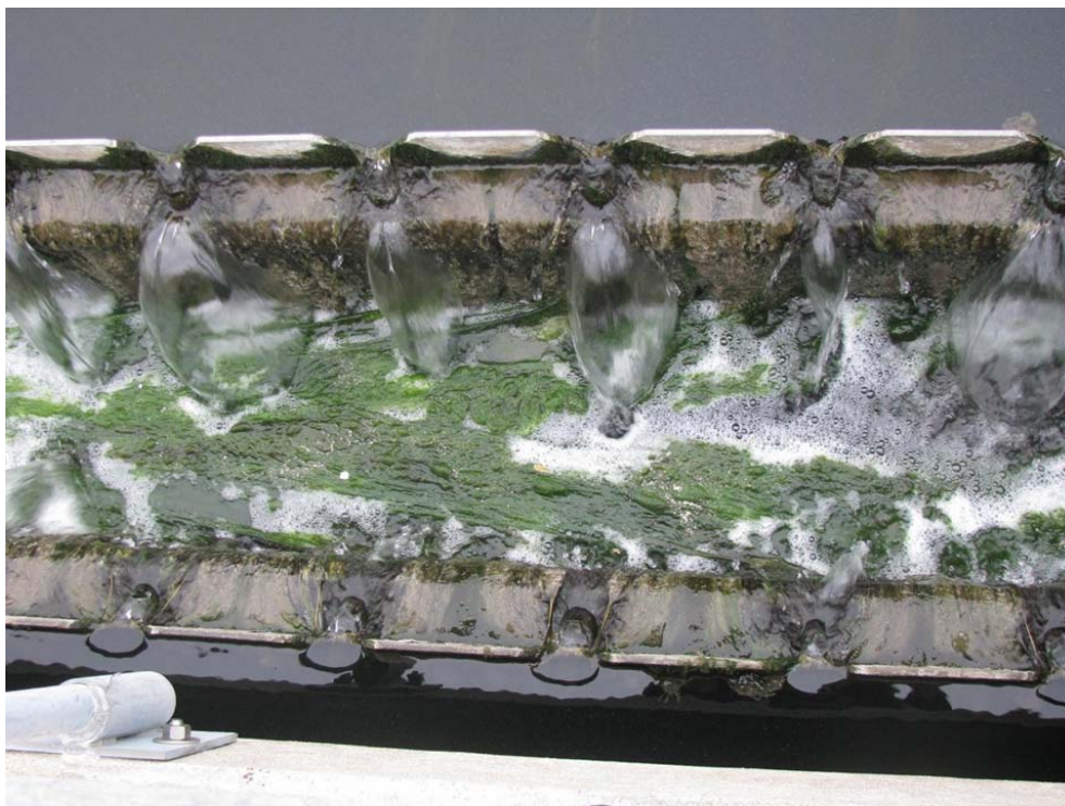
Figure 1. Filamentous algae growing in water treatment plant launders
