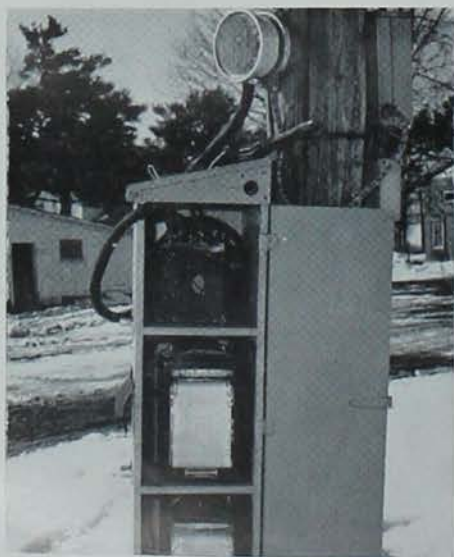
A complicated meter system such as this was installed on each farm being tested for electricity consumption.
