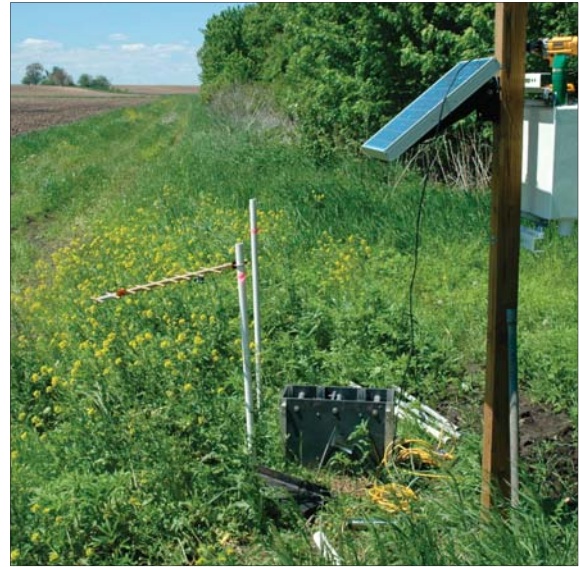
This is where tile water is redistributed. Data is uploaded remotely, powered by solar cells. Credit: Kent Heikens
