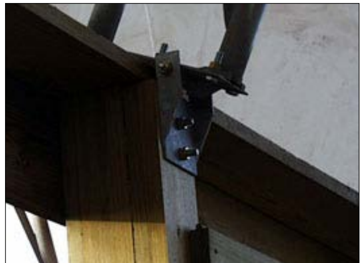
The steel arches are securely fastened to the sidewall to transmit the wind forces to the sidewalls and the ground.
